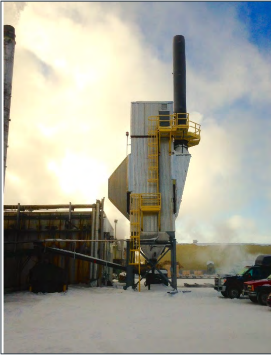
Figure 1: The former plant's electrostatic precipitator
